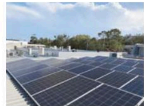
Aspire's solar installation.
