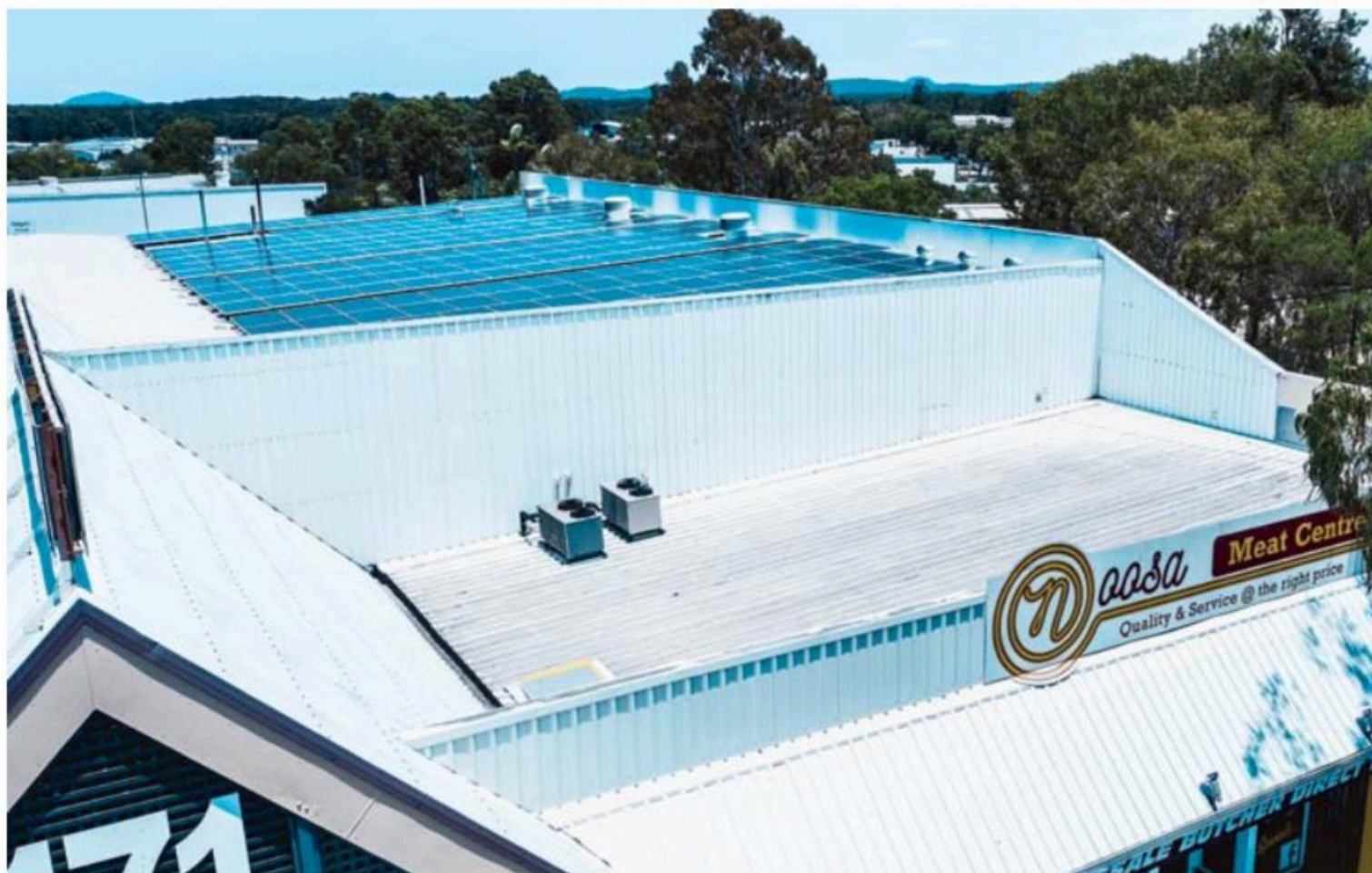
Solar panels at Noosa Meat Centre.
