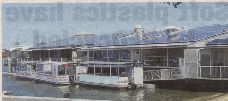
GOING SOLAR: Solar panels on Noosa Marina structures. PHOTO: CONTRIBUTED
